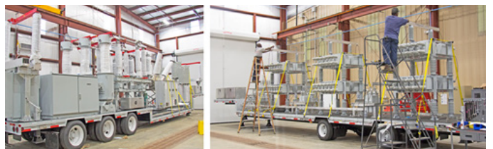
Mobile 115 kV, 550 kV BIL Circuit Breaker & Capacitor Bank Trailer
