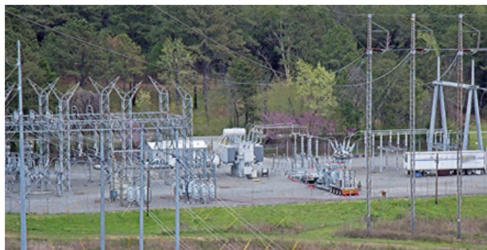
Deployed 35 MVA Mobile Substation 230 kV X 25 kV
