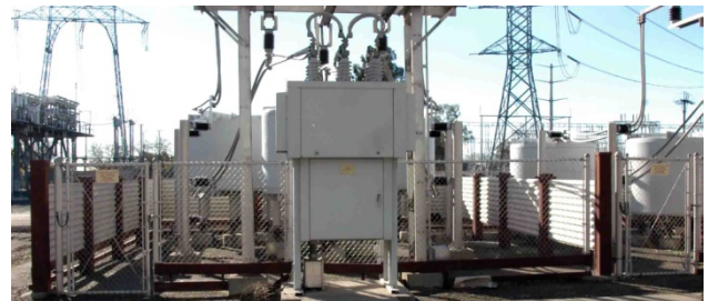
Fig. 7. Air-core dry type shunt reactors switched with a vacuum device
