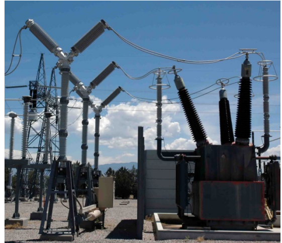
Fig. 6. Shunt reactor switched with a SF 6 breaker
