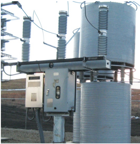
Fig. 10. Special purpose switch for switching shunt reactors
