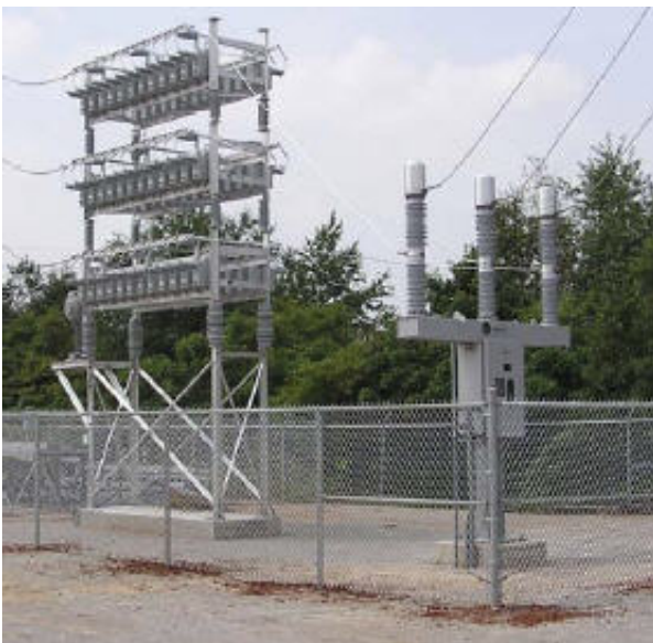
Fig. 14. Shunt capacitor bank with a special purpose capacitor switch
