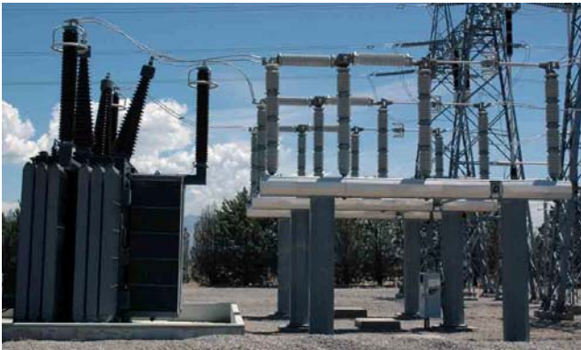
Fig. 8. Oil-immersed shunt reactors switched with a circuit switcher (horizontal interrupter)
