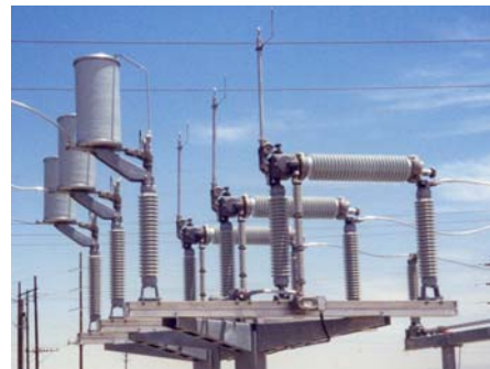
Fig. 13 Circuit Switcher with Pre-Insertion Inductor
