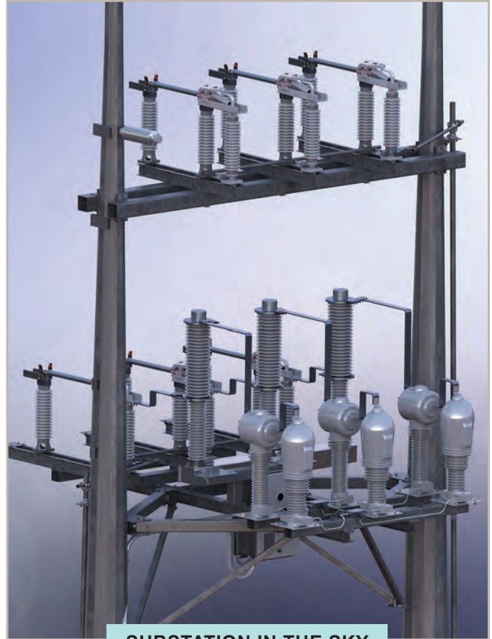
SUBSTATION IN THE SKY
