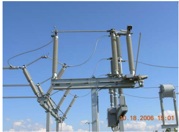
Westhaven Substation (Circuit Switcher w/fault initiating high speed ground switch)
