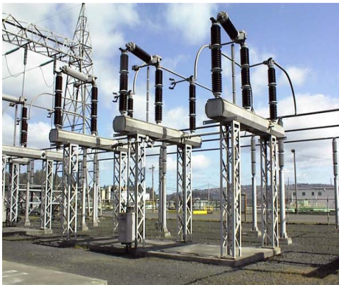
1960's Circuit Switcher Installation
