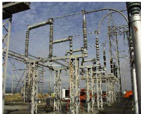
Southern States' Circuit Switcher Installed
