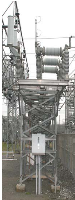
Figure 3 Pre-insertion Inductor Circuit Switcher
