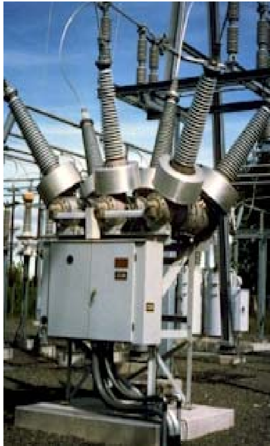
Figure 2 Synchronous Closing Circuit Breaker
