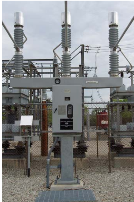
Figure 4 Pre-insertion Resistor Special Purpose Capacitor Switcher
