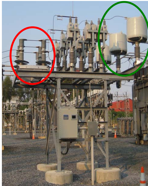
Figure 1 Zero Voltage Closing Vacuum Switch (circled in red) With In-Series Current Limiting Reactor (circled in green)
