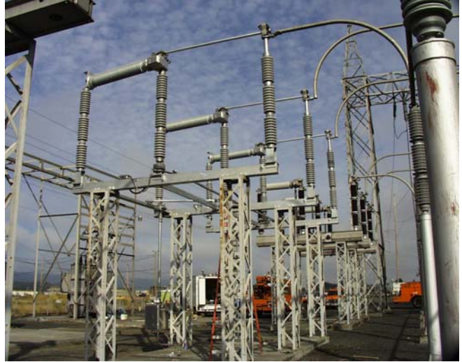
Figure 10 – Shows the Southern States CSH-B circuit switcher that replaced the competitor’s unit and reused the existing structure and foundations
