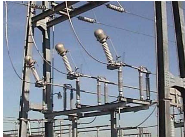
Single Gap Per Phase SF 6 Interrupter On A Vertical Break Switch (1998-2003 Vintage SF 6 Interrupter) Figure 5
