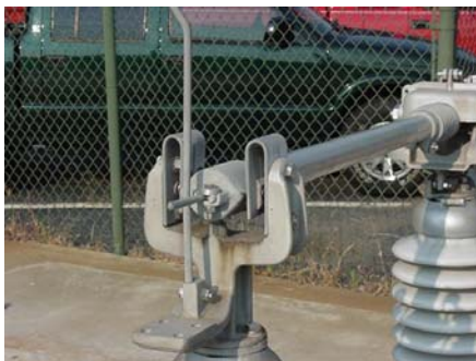
Simple Arcing Horns On A Vertical Break Switch Figure 1
