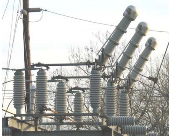
Three Vacuum Bottles In Series Per Phase On A 69 kV Vertical Break Switch
