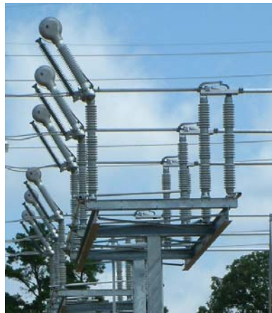
230 kV SF 6 Interrupters With Voltage Limiter On A Vertical Break Switch Figure 7
