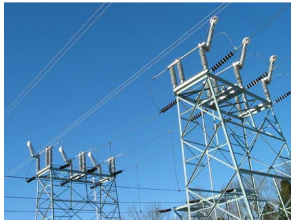
At transmission tap substations, or
